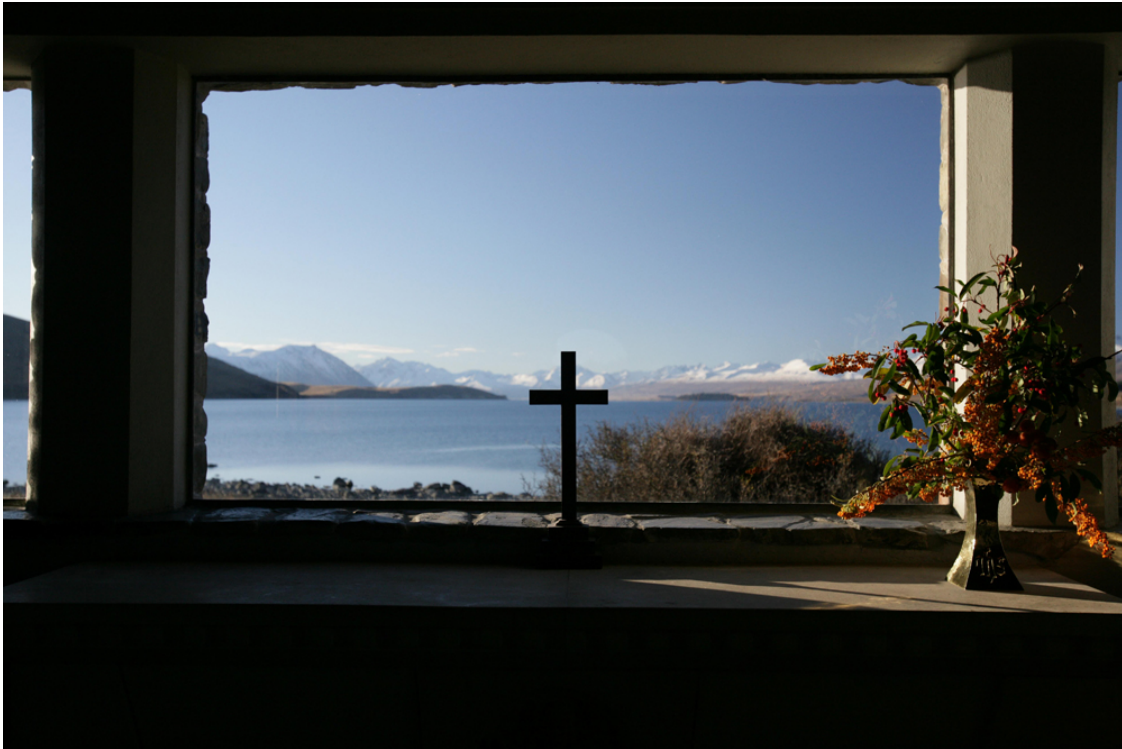
Fig. 11.6. Altar window in the Church of the Good Shepherd, designed “to encompass the beauty of God’s creation”. Photograph: Fraser Gunn
