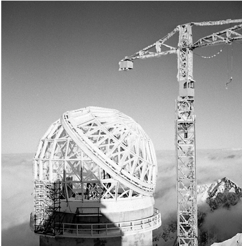
Fig. 9.13. The construction of the dome in 1974. The difficult conditions the mountains are clearly visible: frost covered the buildings and the construction machinery. Photo © Régie du Pic du Midi and Observatoire Midi Pyrénées
